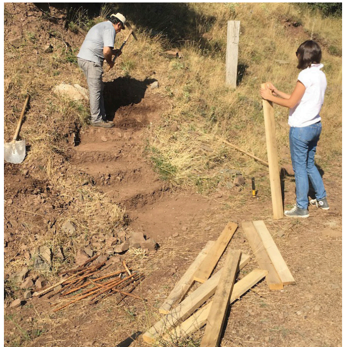
Thanasis Christeas creating a staircase to lead to the hiking trail above the dirt road to the altar of Zeus. Nota Pantzou observes from the road.
