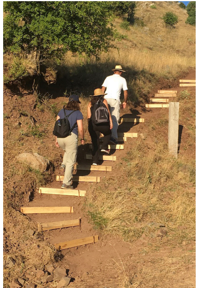
New staircase in use by Catherine Skinner, Fani Kazantzi and John Keck.
