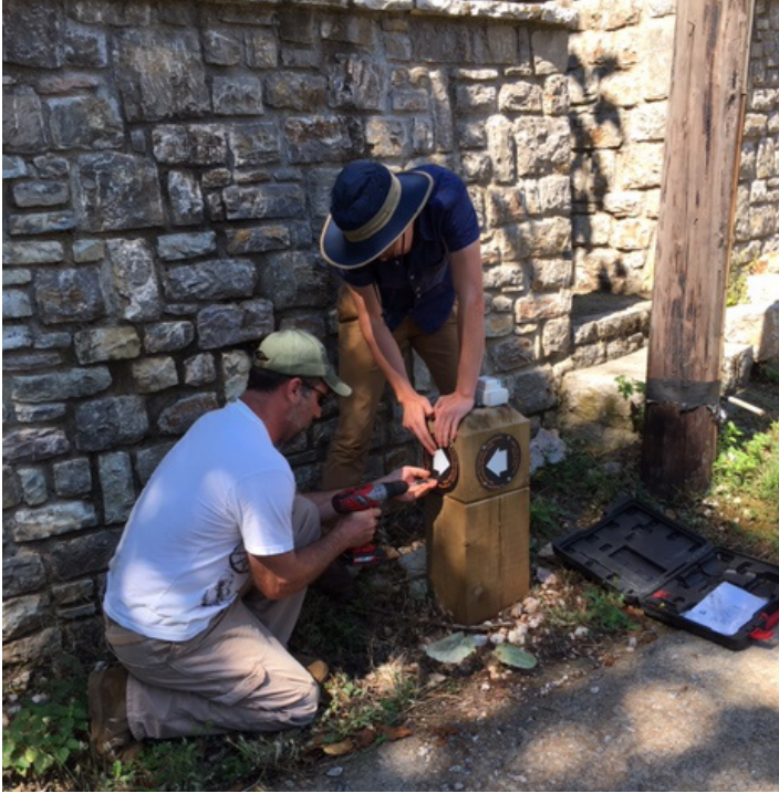
John Keck and Buck Roberson installing a way finding sign for the Trail of Pan
