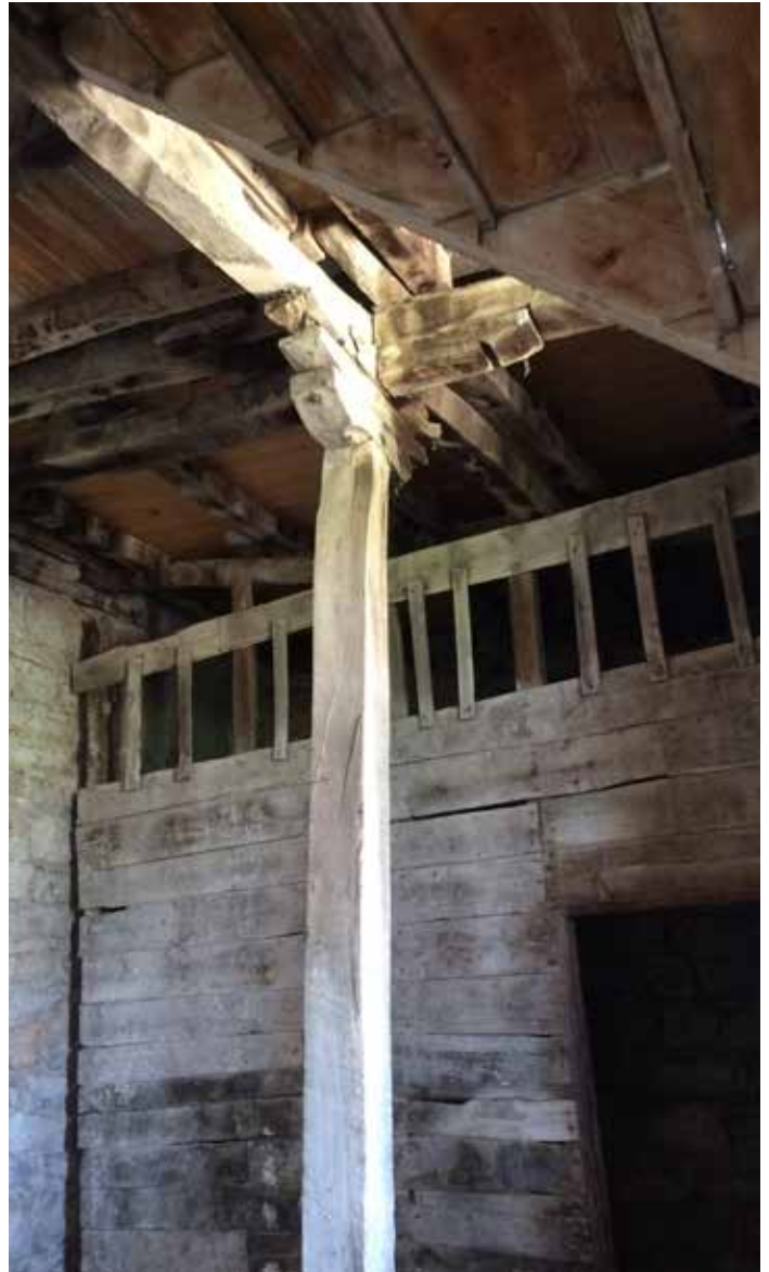
View of interior of basement of the Voyatzis family house. Photo: D.G. Romano.
